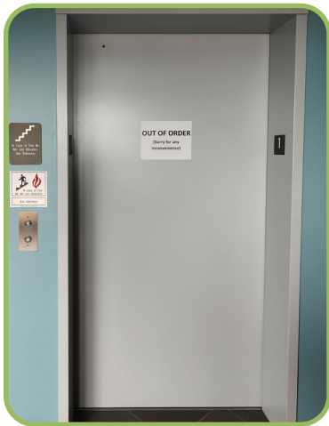
The Spirit Center elevator
